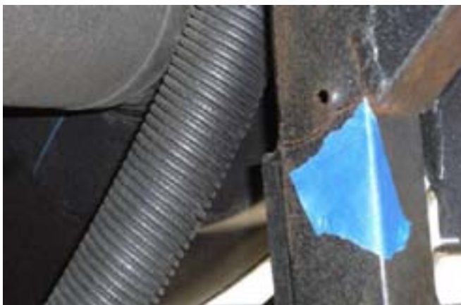
The cracked brace
